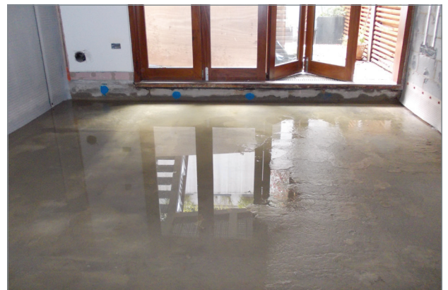
Basement waterproofing failure
