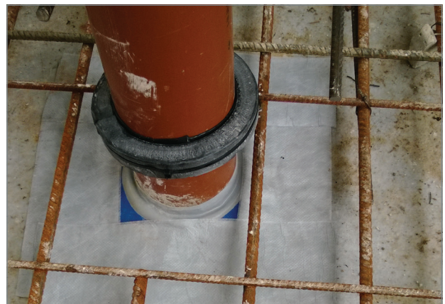
Service penetration flange joint
