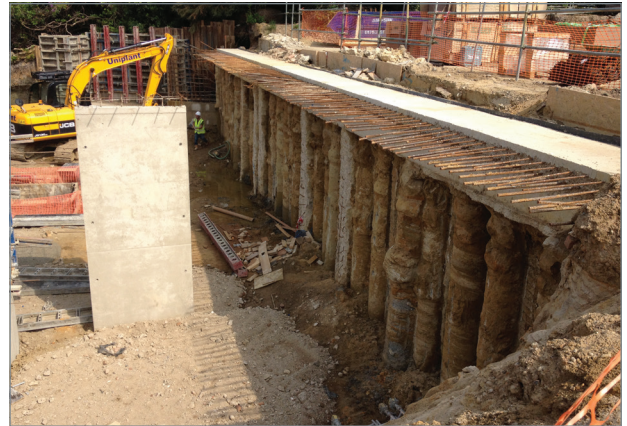
Excavating to basement formation level, secant piled retaining wall to right hand side
